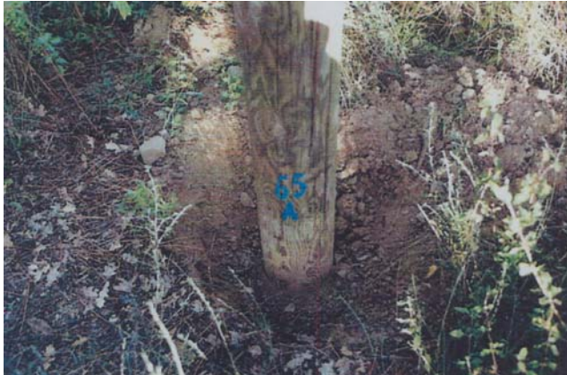
Pole impregnated with CCA after 4 years (Italy)
